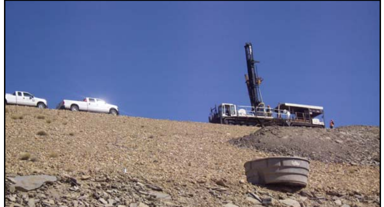
Construction equipment will be returning to the Ritschard Dam at Wolford Mountain Reservoir to install monitoring devices inside the dam.
