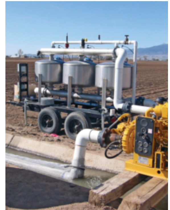
A 2004 CRWCD grant funded this portable drip irrigation system in Montrose County.
