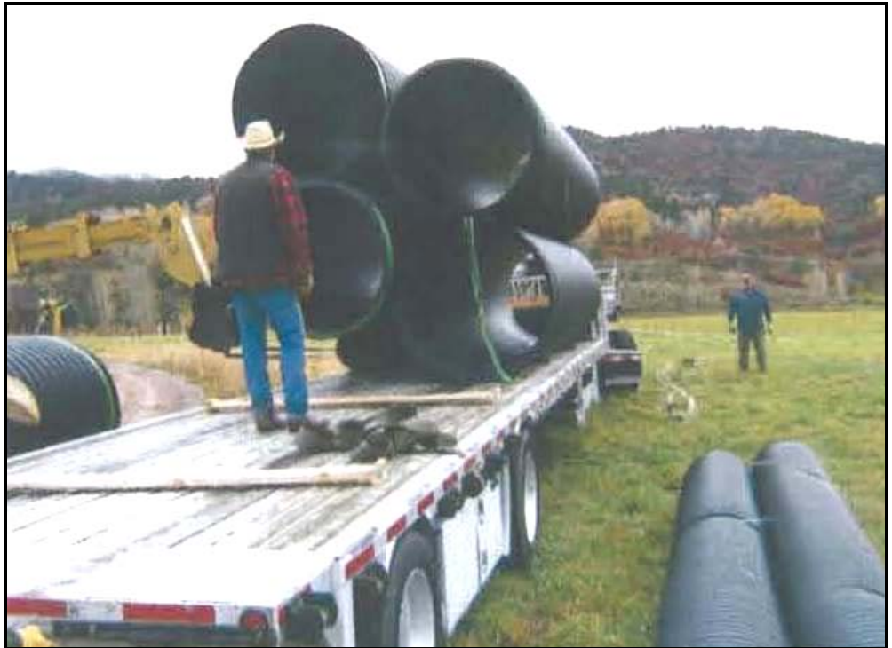
Workmen unload pipe used to repair the East Mesa Ditch in Pitkin County. The Colorado River District awarded $15,000 to the ditch company to assist with the repair of a washout in 2010.
